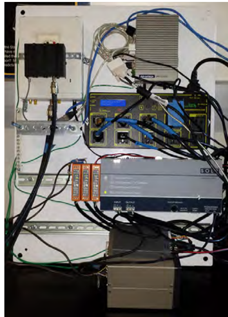
Radio, rotator control and computer system staging and testing for the final design.
