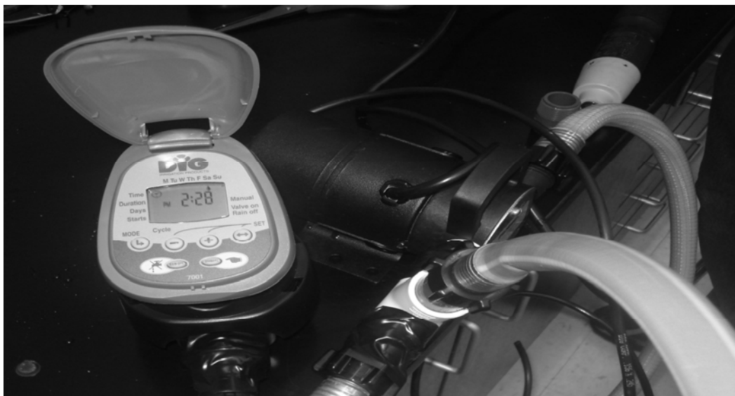
Figure 7 A photograph of the prototype system that consists of a pump, connectors and second timed valve.
